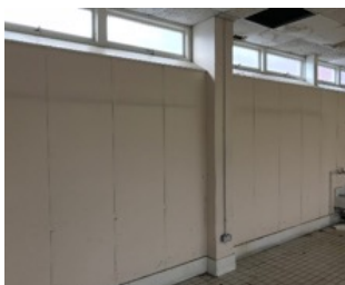
Asbestolux in a wall
