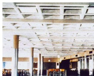
Asbestos spray on ceiling
