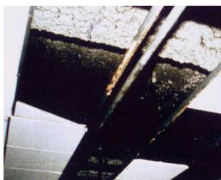
Asbestos sprayed steel beams
