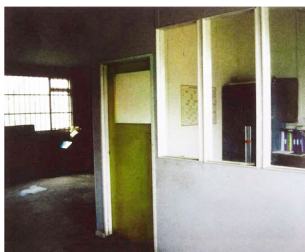
Asbestos insulating boards
