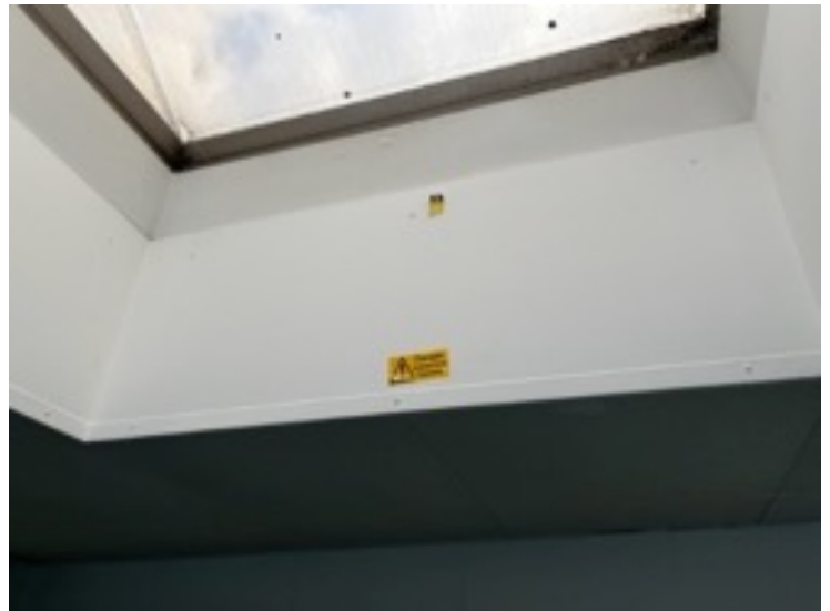
Asbestolux beneath a skylight
