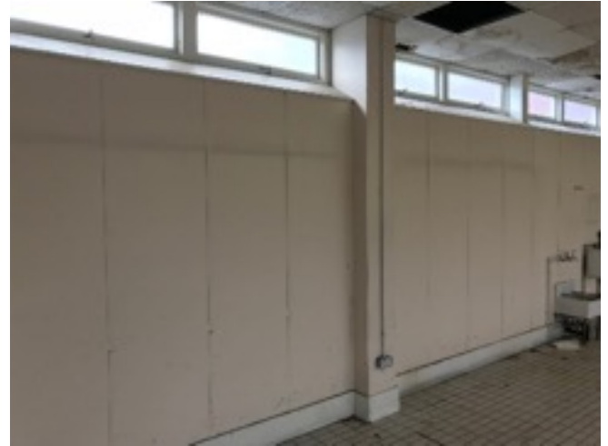
Asbestolux in a wall
