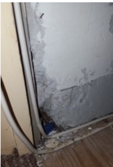
Asbestolux in a wall
