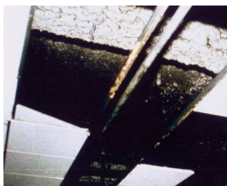
Asbestos sprayed steel beams
