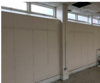
Asbestolux in a wall
