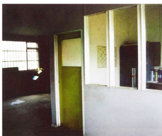
Asbestos insulating boards
