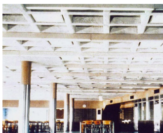
Asbestos spray on ceiling
