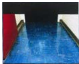
Asbestos floor tiles
