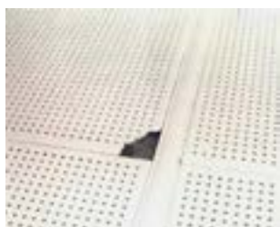
Asbestos ceiling tiles
