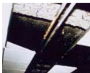
Asbestos sprayed steel beams
