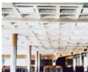
Asbestos spray on ceiling
